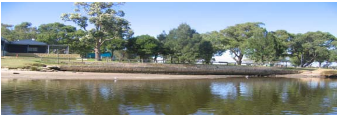
Figure 7.2 Overtopping, lack of drainage management, absence of filter cloth and re-grouting – Qantas Boat Ramp
