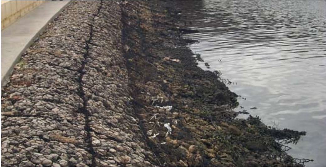
Figure 5.3 Gabion mattresses west of the Narrows, with failure of lower units requiring maintenance
