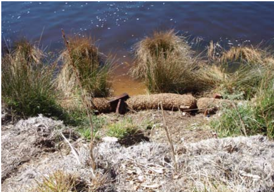
Figure 3.2 Stakes too short
