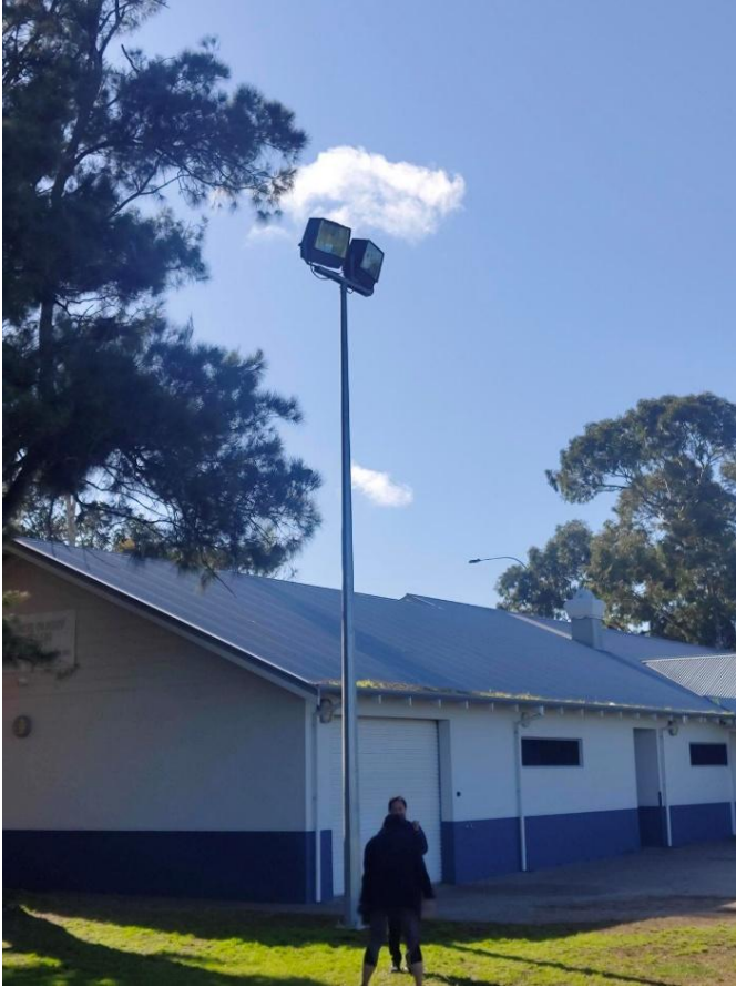
Northern side of reserve at the rugby clubroom, existing light tower (10m high).
