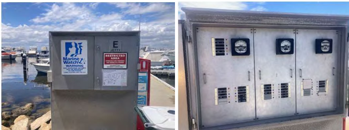
Figure 3.3 Distribution board at E Jetty (existing mains supply for F Jetty)
