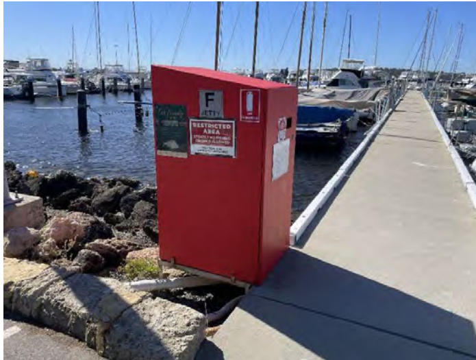
Figure 3.4 Existing Fire Extinguisher
