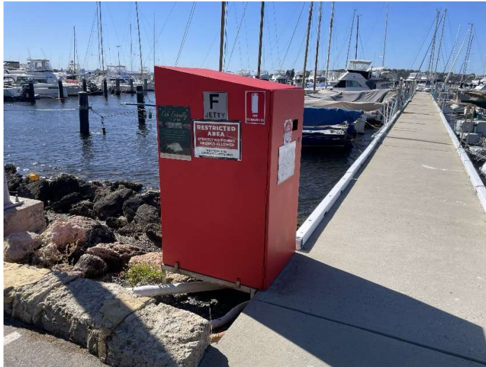
Figure 3.4 Existing Fire Extinguisher (F Jetty example)
