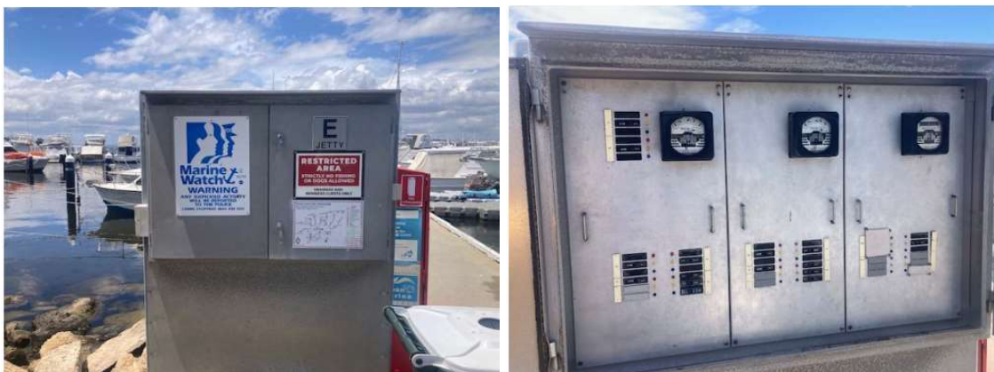
Figure 3.3 Distribution board at E Jetty (existing mains supply for D, E and F Jetty)
