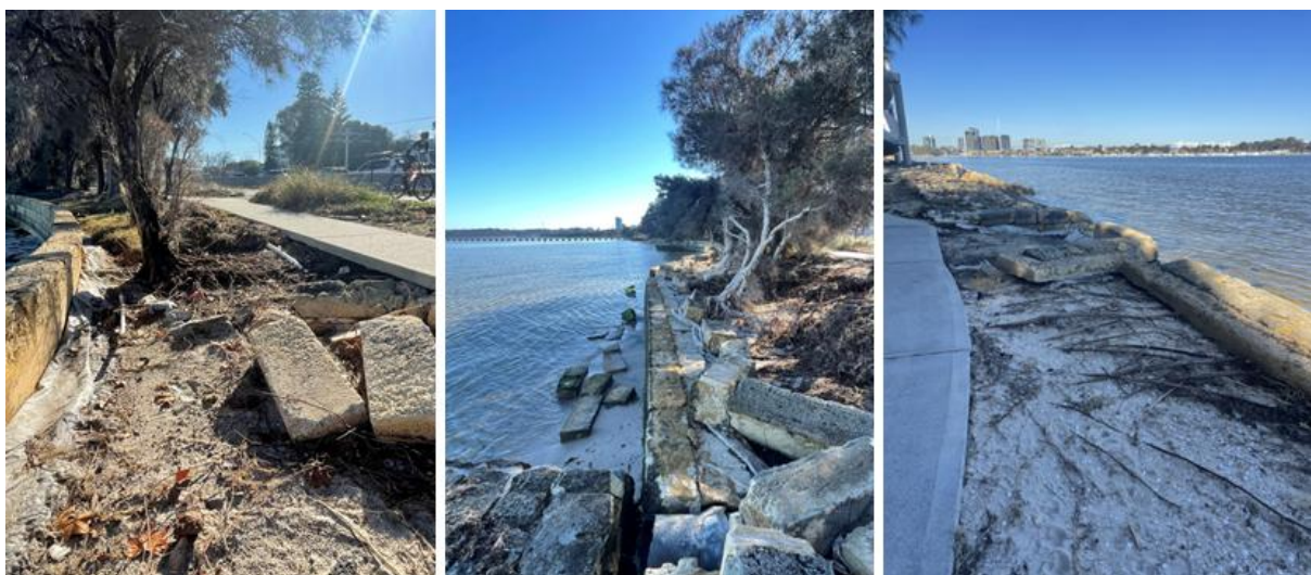
Figure 4-8: Preston Street to Thelma Street – Damaged Limestone Walling
